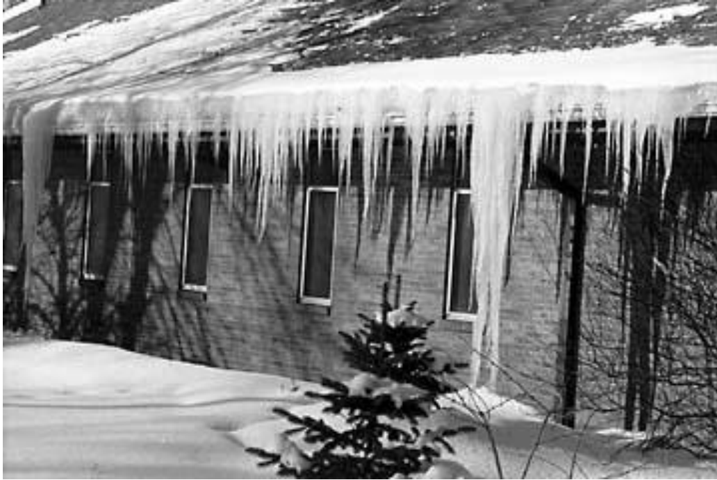
Photograph 2. The unusually high heat loss on this roof has caused both an ice dam and icicles.
