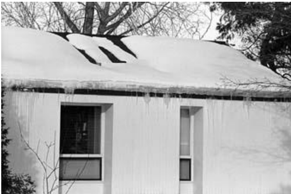
Photograph 1. A single-story house with an ice dam. The areas without snow are the points of heat loss.
