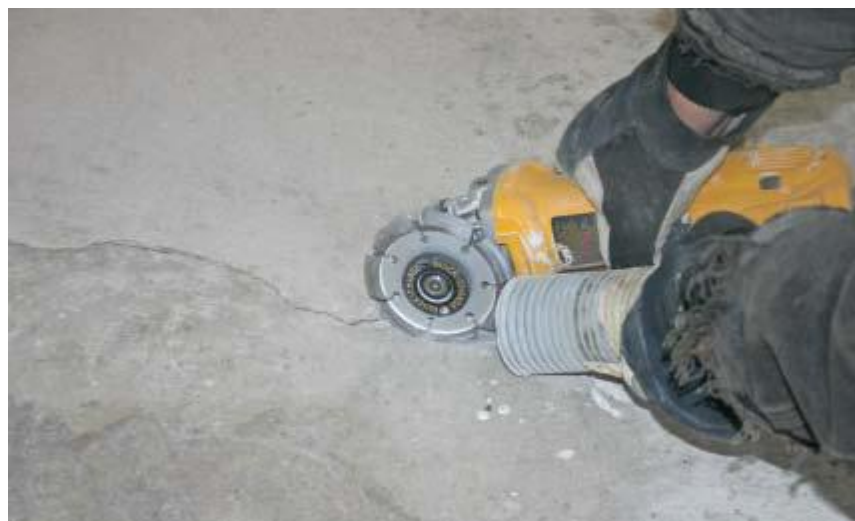
Opening the Crack
