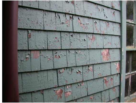
Home built in 1900 – Peeling paint on siding
