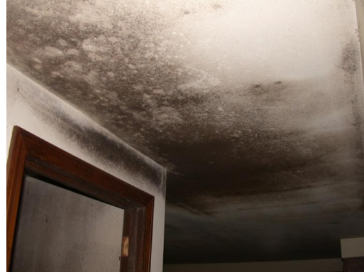
Mid 1960 – mold covered painted ceiling Entire ceiling had to be remove – over 200sqft
