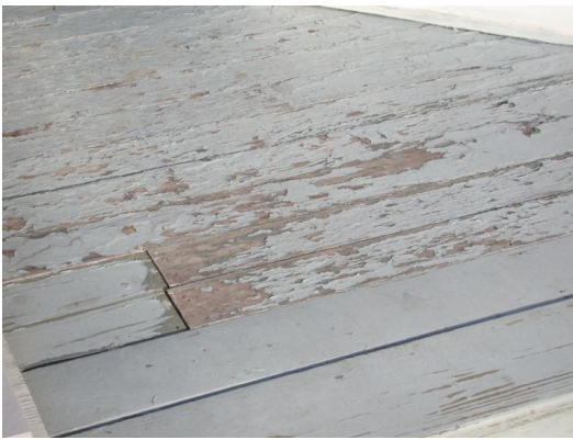
Home built in 1880s - Peeling paint on porch -
