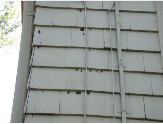
Late 1950s - Damaged siding on all 4 sides –Painted siding Damage was over 80 to 110sqft
