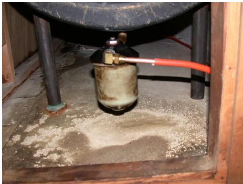
#1-May be a leak from oil filter change
