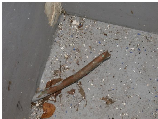
Don't ignore copper tubing coming in from underground!
