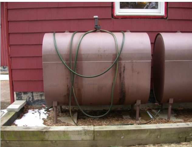
Exterior exposed twin tanks
