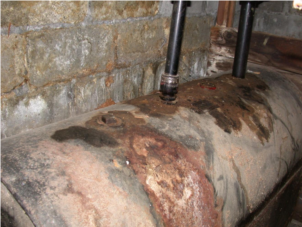
Concealed 550 gallon tank in a basement
