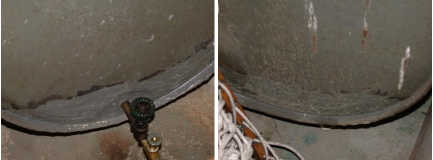
Both sides of this tank were patched.
