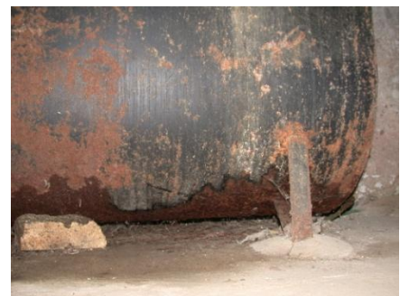
Bottom extremely rusty & damp
