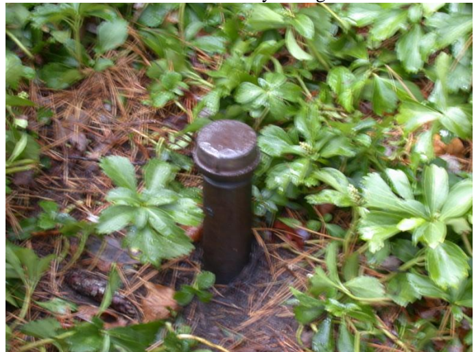
Fill pipe for buried fuel tank in flower bed
